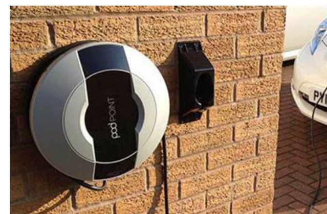
Figure 110: Home electric vehicles charging point example.
