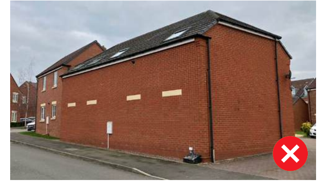
Figure 70: Bricked up windows are unconvincing, with a lack of depth. The large area of inactive facade reduces overlooking and feelings of safety.
